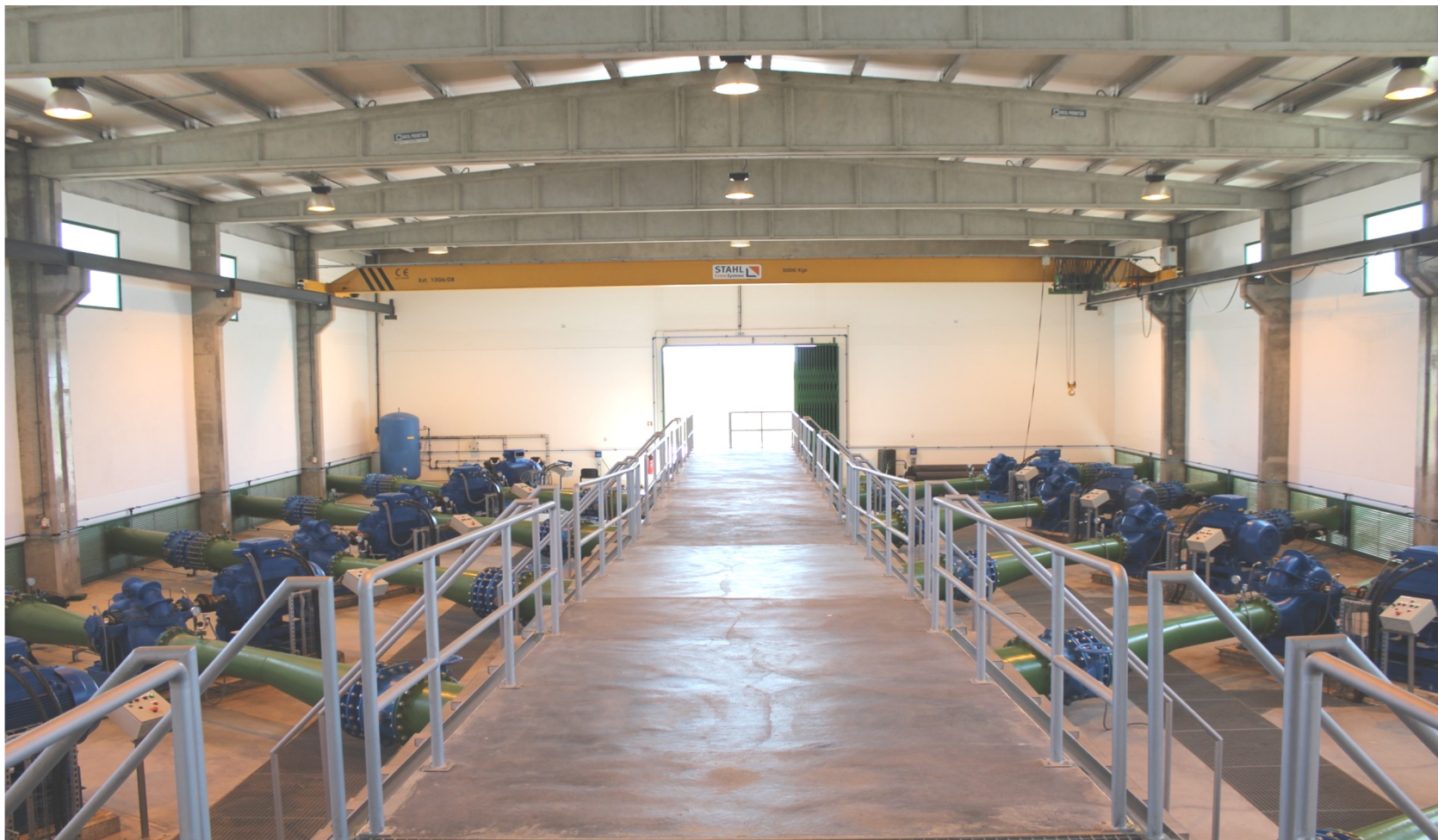
SECONDARY PUMPING STATION
